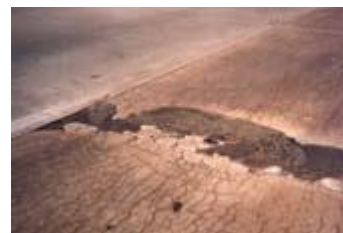
ASR has caused severe damage to this pavement.
