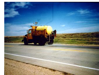
Spraying concrete surfaces is one of three ways to apply Renew® Concrete Treatment.
