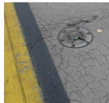
Fig. 1 – ASR Affected airport pavement
